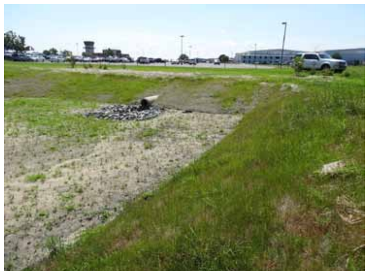
Sand Filter in Wicomico County, MD
